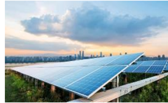
Photovoltaic Solar Panels
