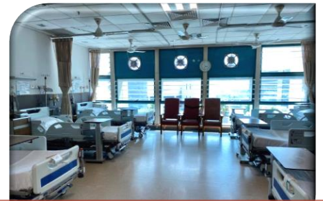
Exhaust fans installed to create negative pressure cohort wards at TTSH Main Building
