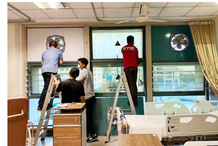
Staff and contracted workers installing exhaust fans as part of the ward conversion efforts – turning BAU Wards into COVID-19 Wards at TTSH.
