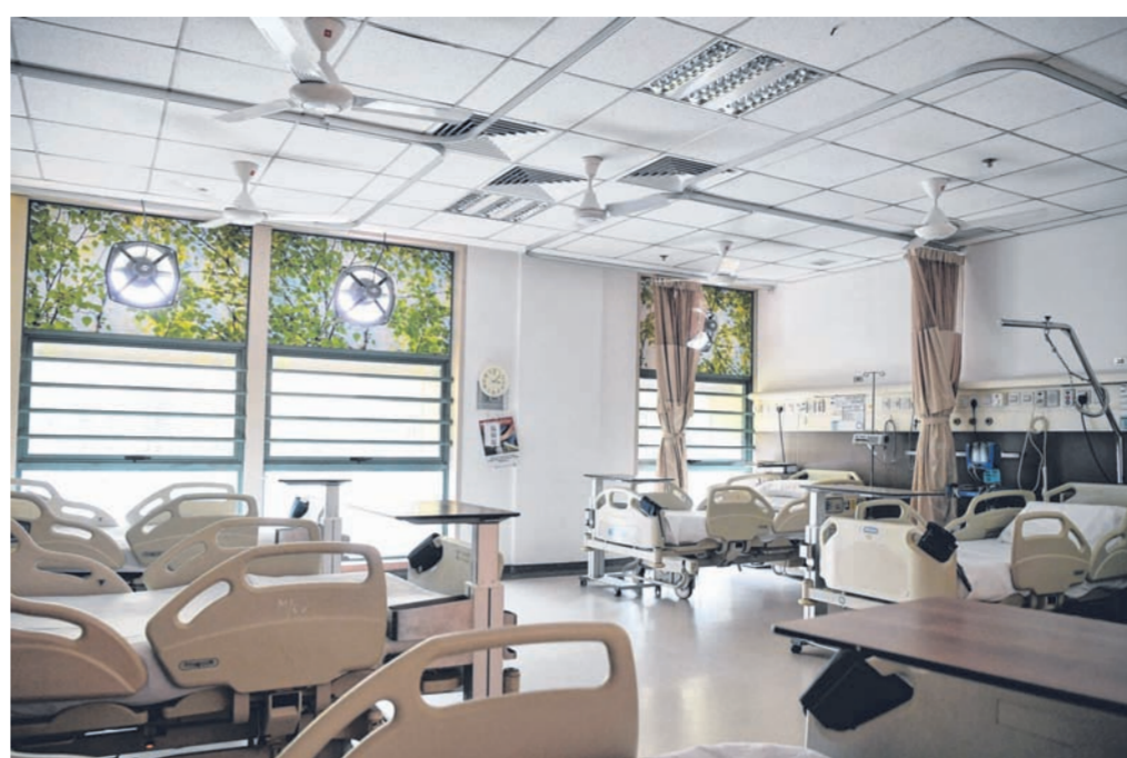
Exhaust fans installed at the windows in a Covid-19 ward at Tan Tock Seng Hospital. They draw out the air and create constant ventilation. ST PHOTO: KUA CHEE SIONG
